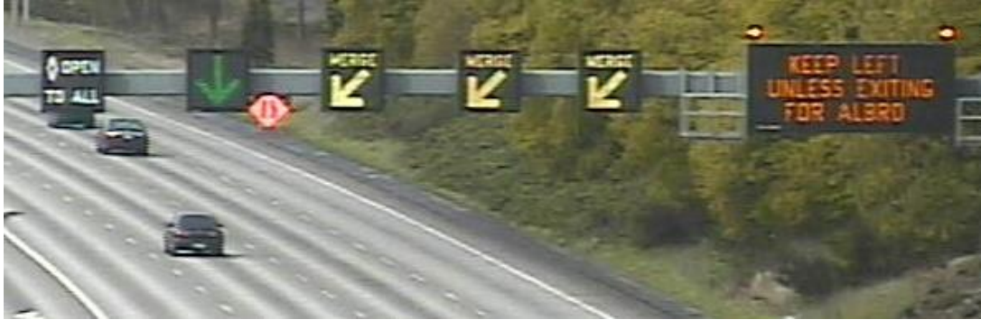
Figure 3: ATM Lane Use Control Signage on Northbound I-5 in Seattle (Source: WSDOT)
