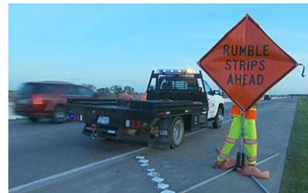
Queue Warning System in Texas incorporates temporary rumbles strips
