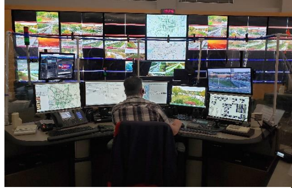
Figure 5: Curtains from PVC pipes around MnDOT RTMC Workstations Photo Courtesy of MnDOT
