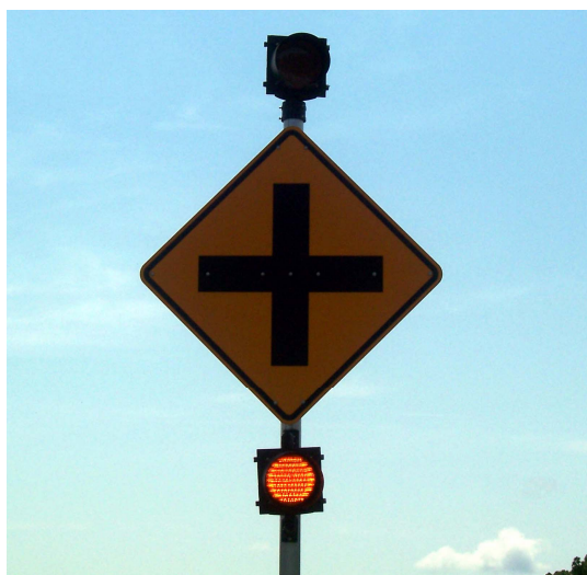
Figure 13 Example Vehicle Actuated Advance Warning Beacons
